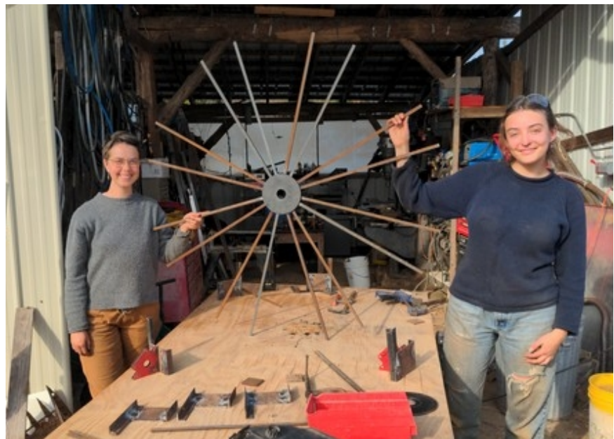
Ayla and India are volunteers at LEF. We taught them to weld, and they are building our peristaltic pump for the biogas digester.
