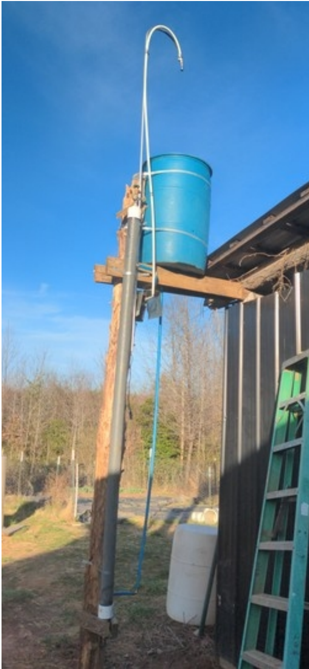
Biogas filtration tower. The grey pipe is the bubbler section. The water is pumped up to the showerhead over the blue barrel. CO 2 is dissipated into the air, and the water recirculated.
