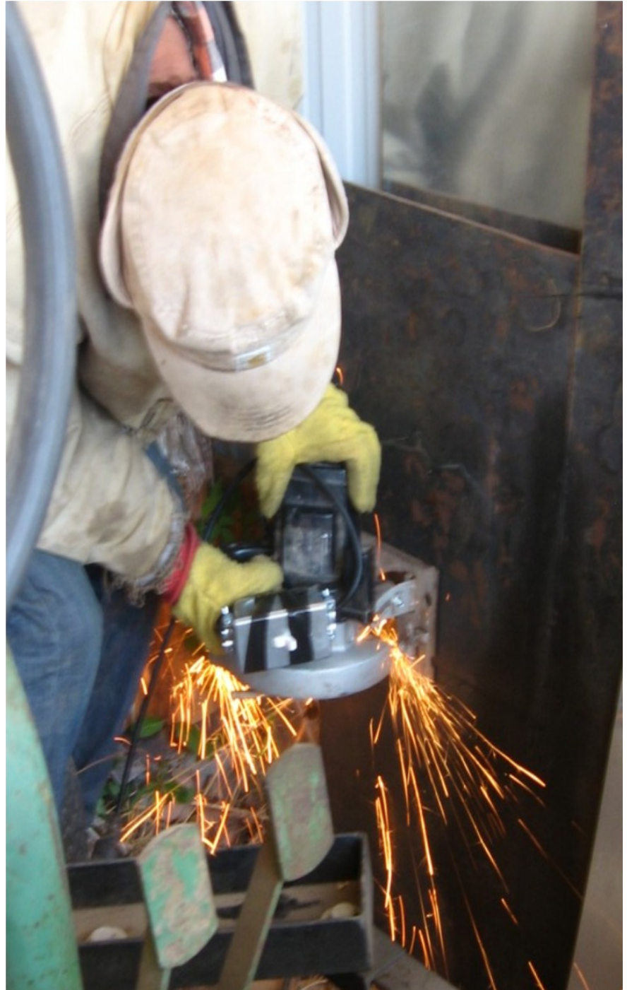
Alexis cutting quarter inch plate steel with a circular saw powered by daylight drive solar electricity. DC electricity is powerful!
