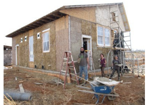
Sean, Al and Carrie apply stucco over the straw bale kitchen walls..
