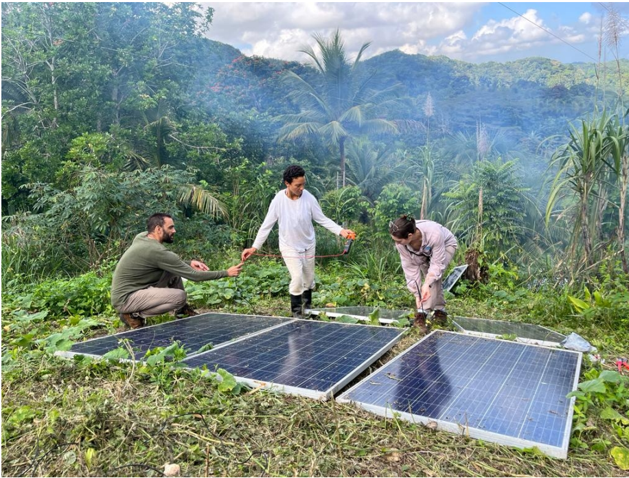
Ricardo, Millo, and Marielisa from Puerto Rico helping out installing direct drive solar DC equipment in Jamaica.
