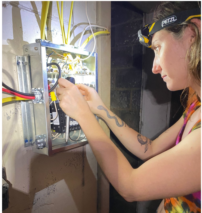
Marielisa wiring a low voltage DC distribution center.
