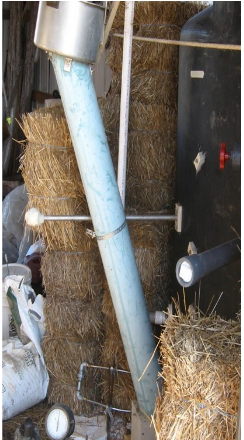
The new biogas digester being entombed in not one, but two layers of strawbales. The secret to biogas is to keep the digester very, very warm (and feed it every day).
