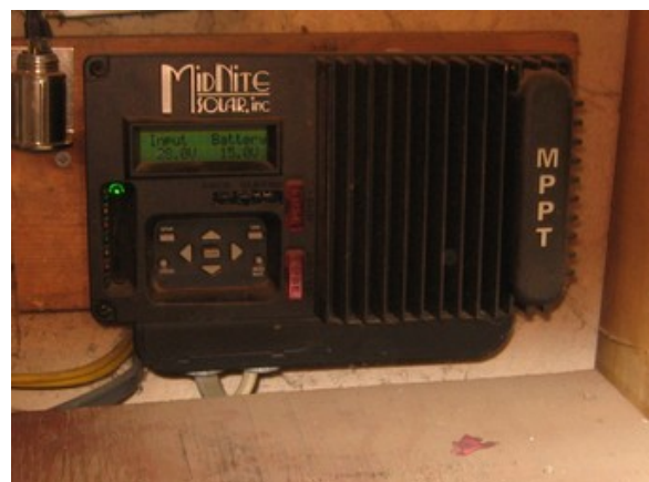
This is a $350 MPPT controller at LEF. One can also use a $90 controller if nominal 12 volt panels are used.
