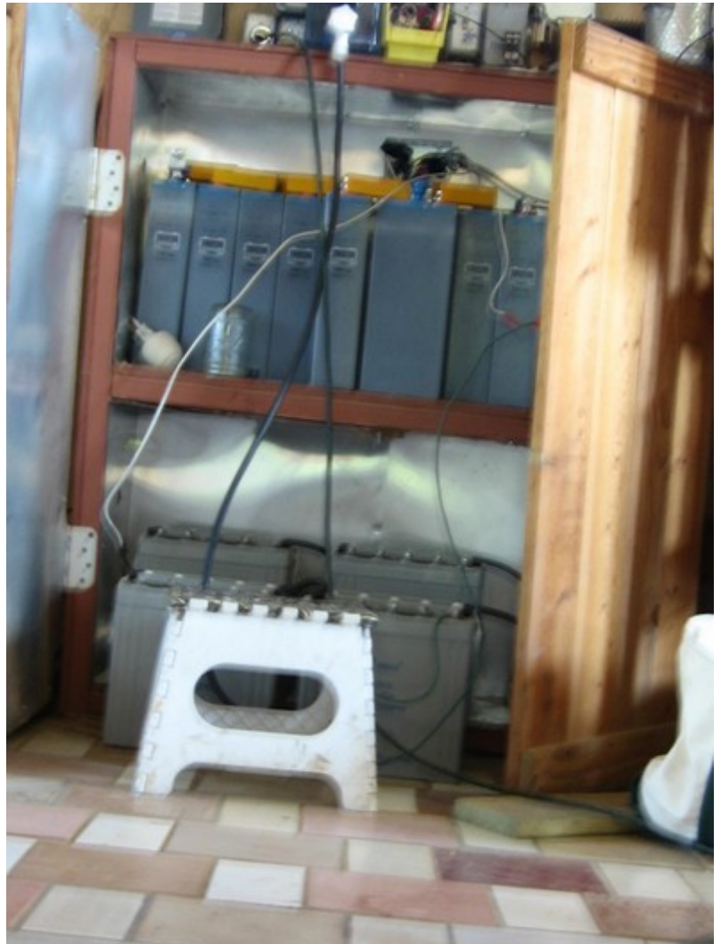
Nickel iron batteries undergoing endurance testing.
