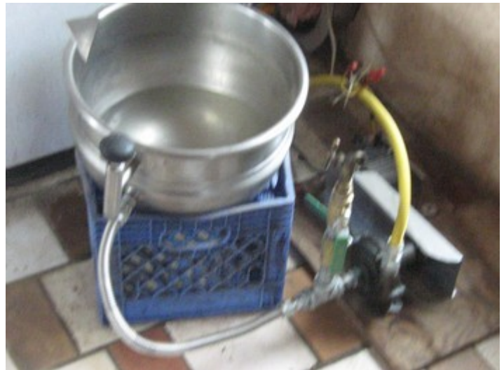
The indoor part of the solar high temperature cooking system, a steam jacketed kettle and a DC pump. It gets hot, but not hot enough.
