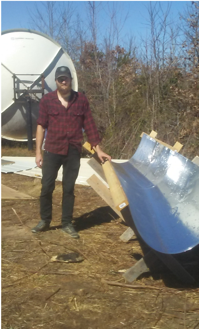
Eddie starts work on the tropical solar boiler, the cold-weather hardware in the background.
